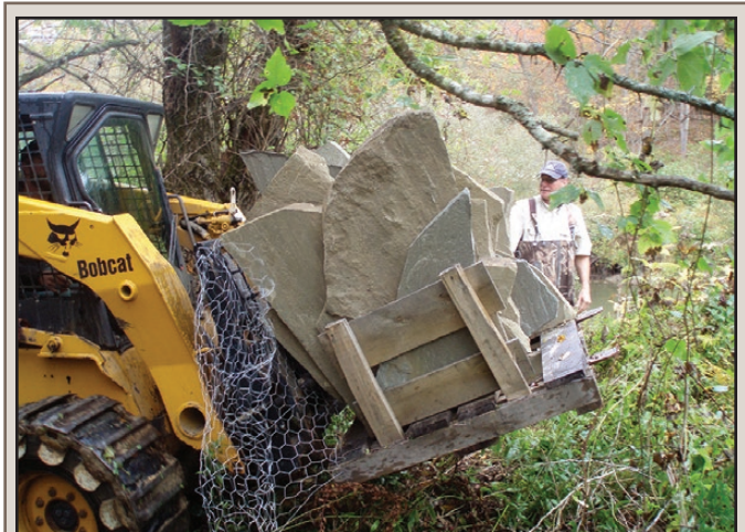
FIG. 1. Skid steer hauling flagstone cover rocks down to enhancement site where they were hand placed.
